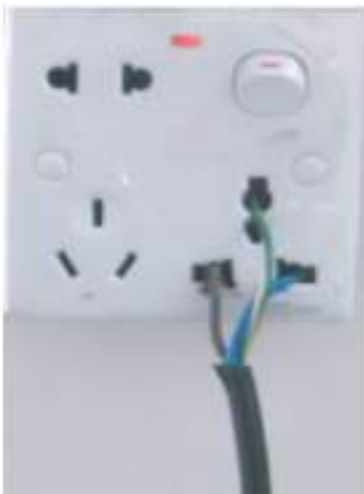
Risky electric connection
